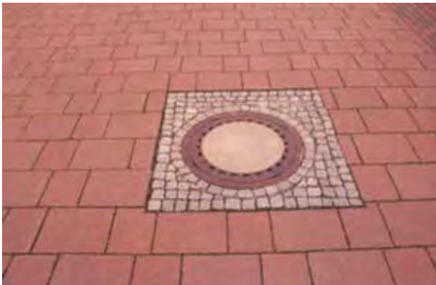
Figure 29. Filling the outside of a utility cover with mortar-set stone paving units
