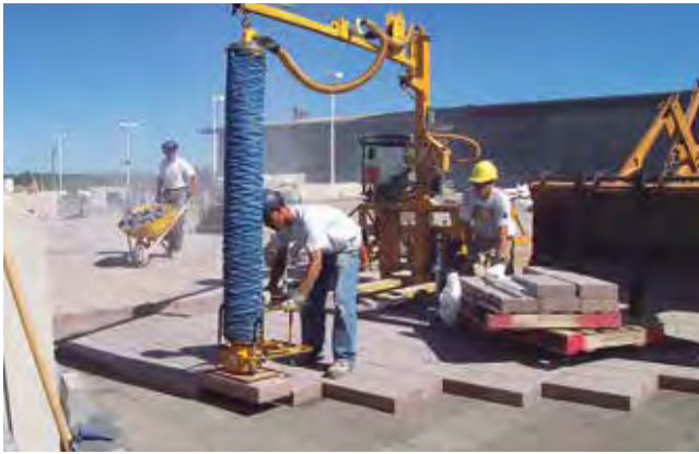
Figure 12. Self-contained vacuum lifter with boom
