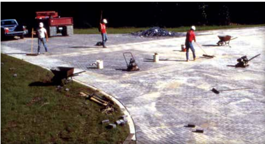
Figure 12. Removing excess sand from the finished surface will make the pavement ready for traffic.
