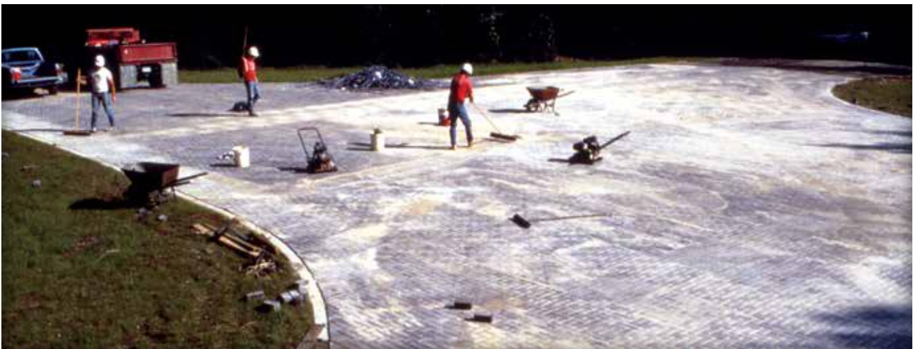
Figure 12. Excess sand swept from the finished surface will make the pavement ready for traffic.
